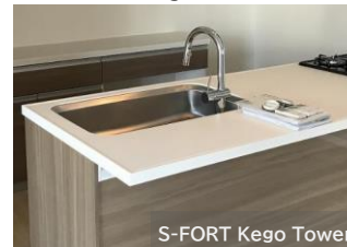
<Introduction of touchless water-saving faucets>
